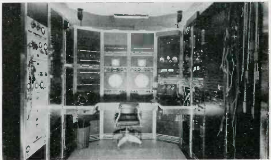
WNBT-W2XWG CONTROL ROOM of NBC "uhf center" at 85th floor of Empire State Building, New York City
